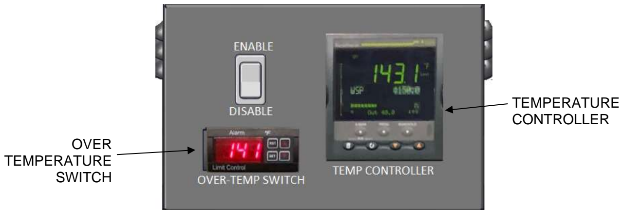
Figure 8.3.3-1. Over-Temperature Switch & Temperature Controller
