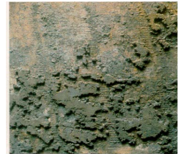
UNDER DEPOSIT CORROSION
